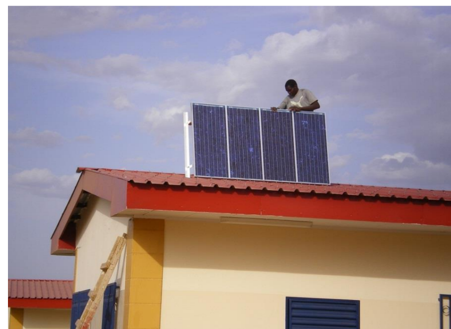
Installation kits SOETAP - RDC 2010
